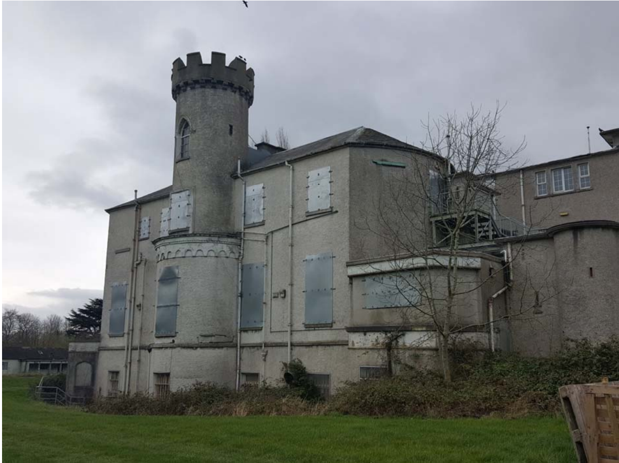
Image 13.55: The abutment of the 1950s block to the original building is clearly noted from the north-east.
