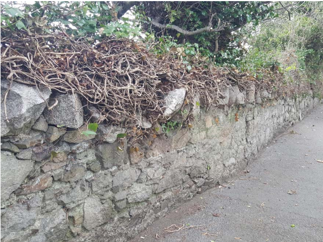
Image 13.36: Rubble limestone boundary walls on the western side of the road, across from the development site and in the vicinity of the development remain as an important part of the historic public realm, along with mature trees, hedgerows and shrubbery that create a close envelope edging the public paths and support the sylvan character of the Dublin Road.
