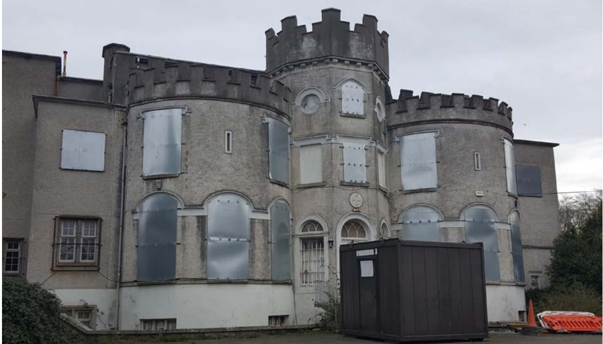
Image 13.48: Front (south-west) elevation of Shanganagh Castle, developed c.1765 and altered by Sir Richard Morrison c.1805-1818. (RPS ref. 1845, RMP ref. DU026-120, NIAH ref. 60260146).
