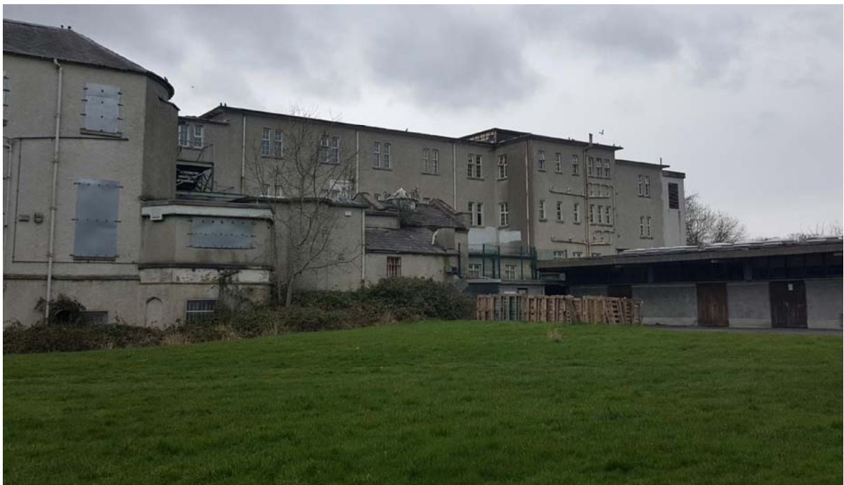
Image 13.52: The 1950s three-storey block is located to the north and is of poor quality.
