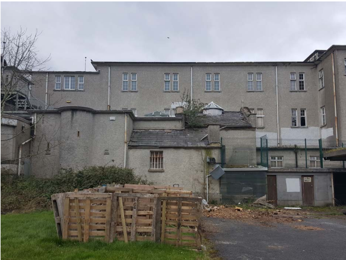
Image 13.54: The low-lying extensions to the rear of the castle and of the 1950s extension are in poor condition. Some of these elements date to Morrison's refurbishment of the 18th century castle, whilst others are 20th century interventions.
